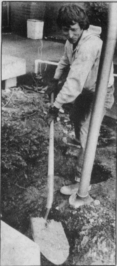
An S.U. maintenance worker digs for a broken water main outside Connolly Center.
