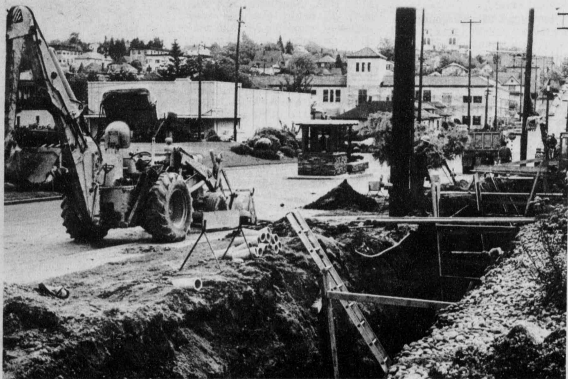
CROSS OVER THE BRIDGE: Construction of a steam line from the main campus to the Physical Education Center has created a moat effect to the front of Bellarmine Hall. Large ditches in front of the dorm are covered with plywood bridges. Spectator Photo by Don Conrard
