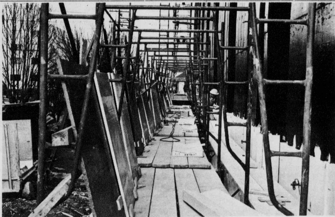
DECORATIVE ADDITION: Scaffolding surrounds the new A. A. Lemieux Library in preparation for the placing of marble which will face the structure.
